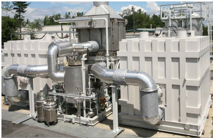
SureSource3000 2.8MW Powerplant
